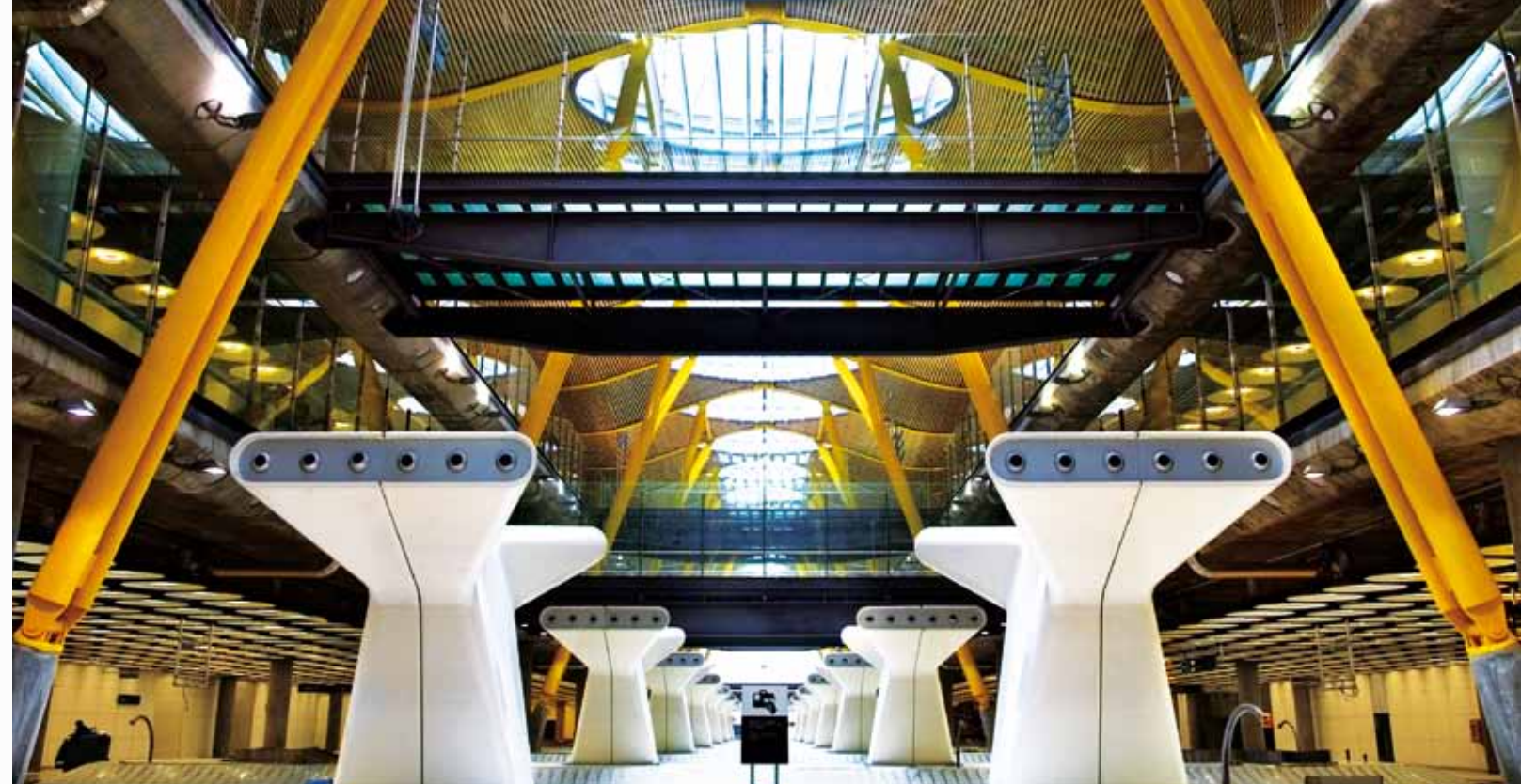
Integrated approach: ventilation components, like the TROX jet nozzles shown here in the baggage handling area, are an integral component of the architecture.
